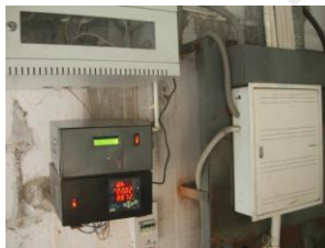
Fig.10 Meter Installed at Palit building's incomer
