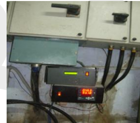
Fig.9 EM Installed at Departmental incomer
