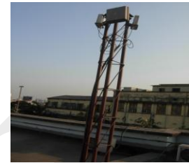
Fig.6 Antenna MAST at Departmental Rooftop
