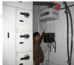
Fig.12 Meter Installed at College street Campus's incomer
