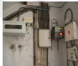
Fig.11 Meter Installed at PG Hall's (men) incomer
