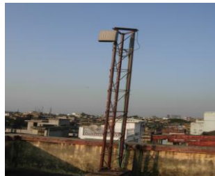
Fig.4 Antenna MAST at PG Hostel
